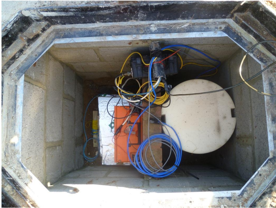
Figure 1 View into the seismic well, showing the Guralp seismometer encased within a foam box to minimize the effects of air circulation on the instrument. The data logger and model is contained with the black Pelicase. 12 v power and communications are provided via a buried conduit to the lamp-post adjacent to the site, which is seen entering the well at the top of this photo.
