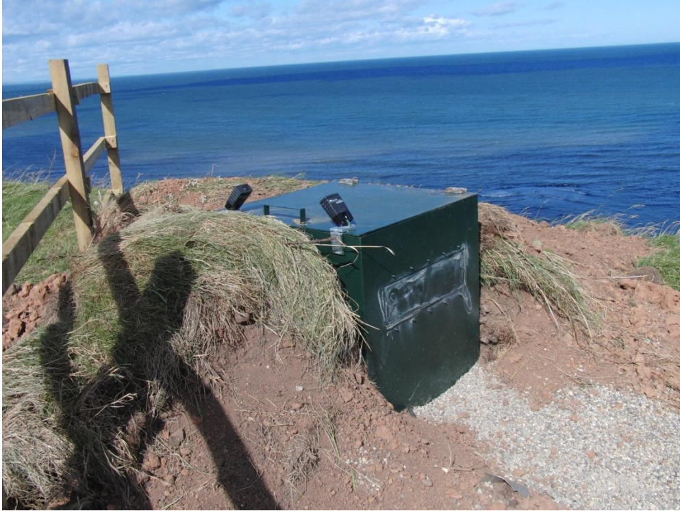
Figure 13 View of the automatic window (closed) on the scanner housing.
