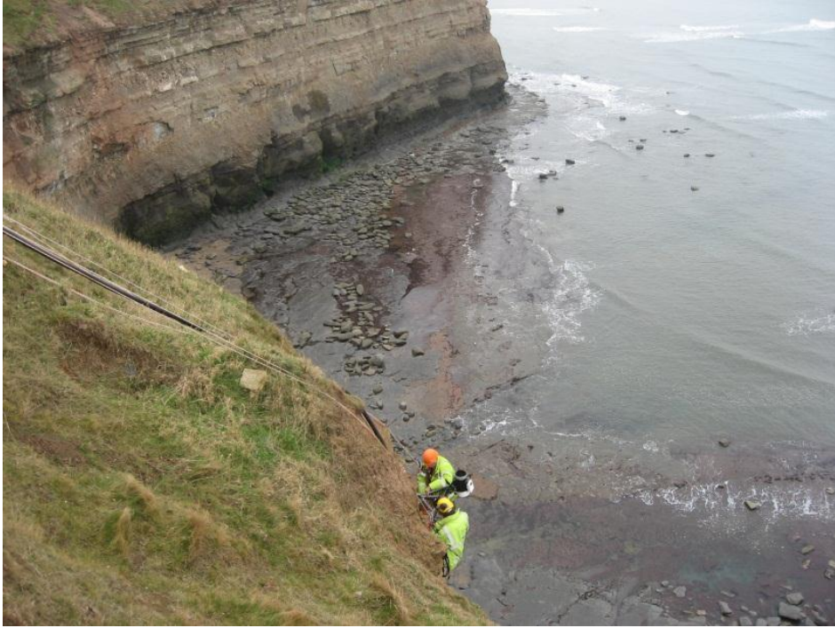
Figure 6 Installation of the cliff face instrumentation, including weather station, laser radar and camera.
