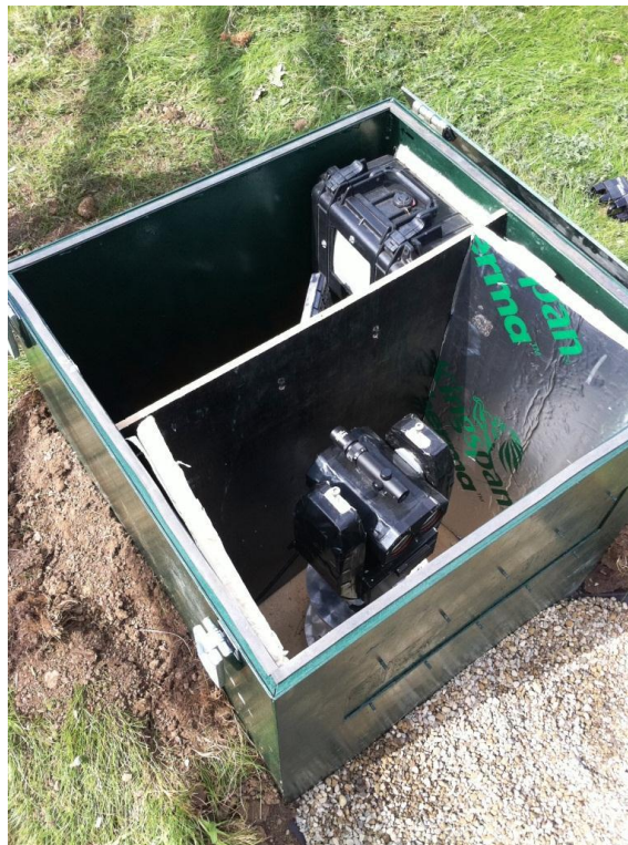
Figure 12 View inside the permanent scanner installation, showing the scanner nearest to the window mechanism, and the controls PC at the rear of the box
